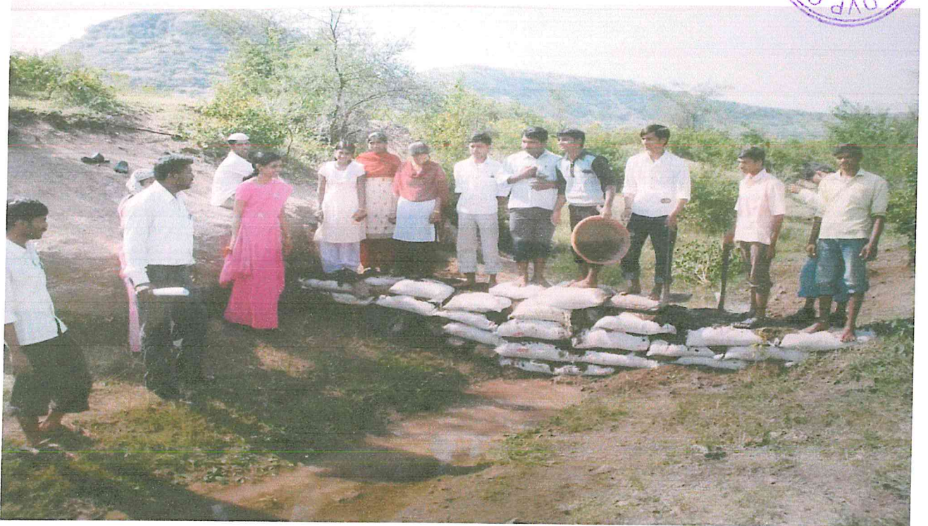
Water Conservation- NSS volunteers made a dam with bags of sand and soil
